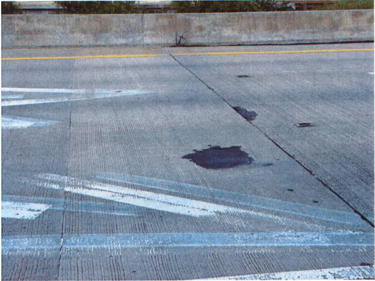
Pic. # 32 Asphalt Patches at the Abut 2 side of Bridge # 19-I440-4.36 R
